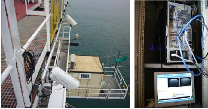
Figure 2: (Left) deployed WASS at Acqua Alta , and (Right) workstation and cables.
