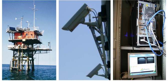
Fig. 1. (Left) Offshore platform “Acqua Alta” in the northern Adriatic Sea, near Venice. (Center) Pair of synchronized cameras for monitoring the ocean climate from the platform. (Right) WASS hardware installed at the platform for recording stereo videos of ocean waves.
